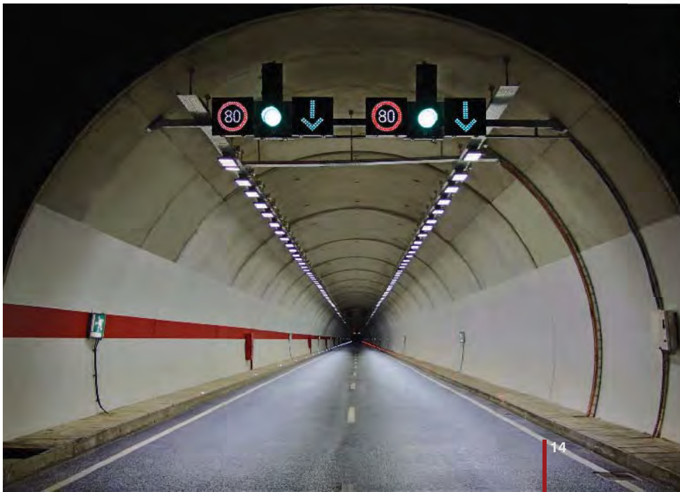
Gumushane Tunnels, ITS Project / 2017 Gümüşhane Tunnelleri, AUS Projesi
