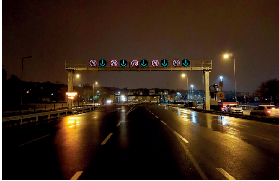
İstanbul Eurasia Tunnel, VTS / 2016 İstanbul Avrasya Tüneli, VTS
